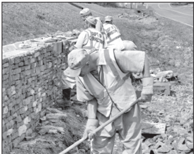
County detainees worked for a week to put a new face on an existing retaining wall near the recreation center
